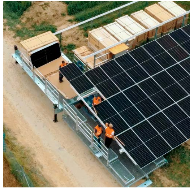
MONTAGE 2.0 in action: The installation of the PV modules is done from the side – they are pushed on as a 'whole table' on rollers.
